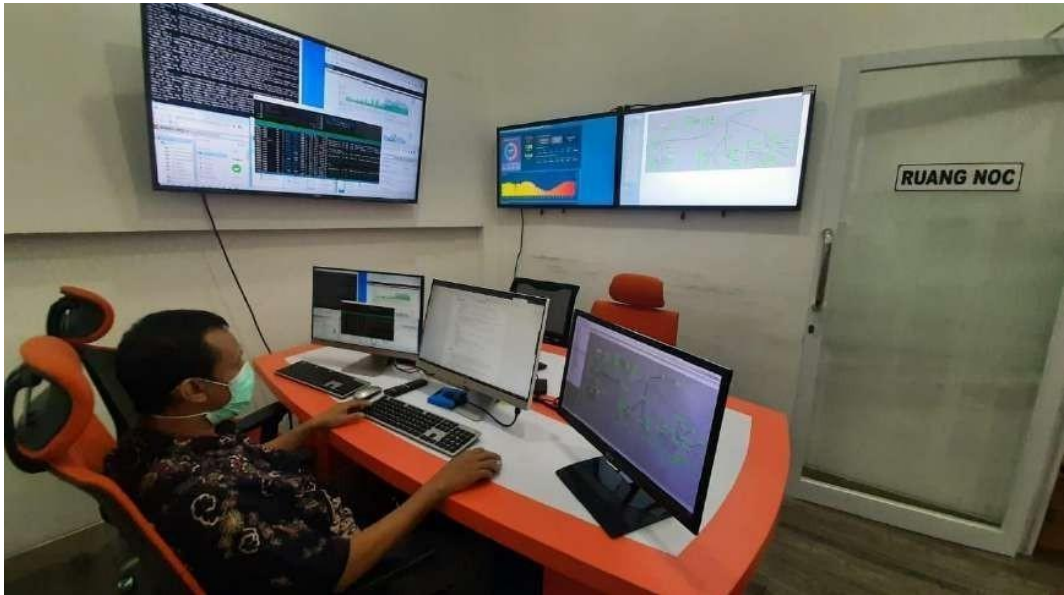
Gambar 2.9 Ruang Network Operation Center (NOC)
